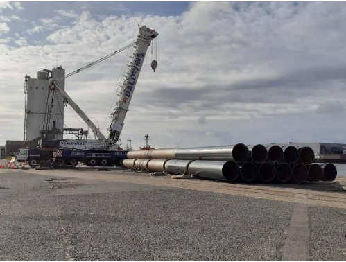
Dolphin Piles – North Quay
